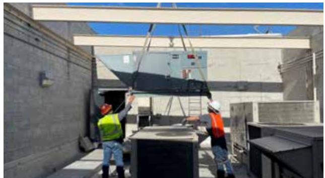
Managed the replacement of the HV unit at the Anaheim Bus Base Operation Building, including roof and structural work.
