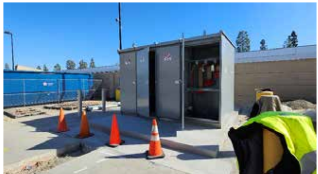
Managed the Installation of the 12kV switchgear equipment project at the Santa Ana Bus Base.
