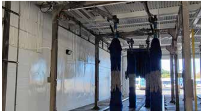
Oversaw building repairs at the Garden Grove Bus Base wash building, including roof repairs and high-performance coatings.
