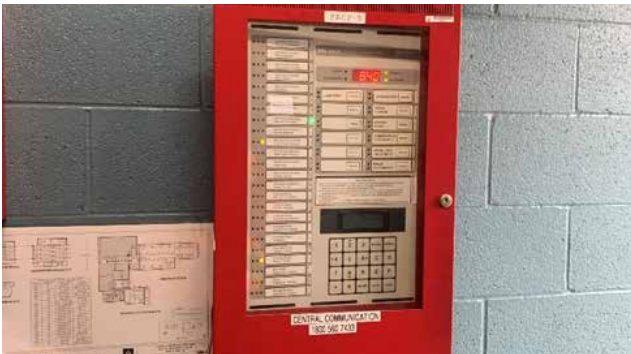
Managed the replacement of this outdated fire alarm panel that controls several buildings at the Santa Ana Bus Base.
