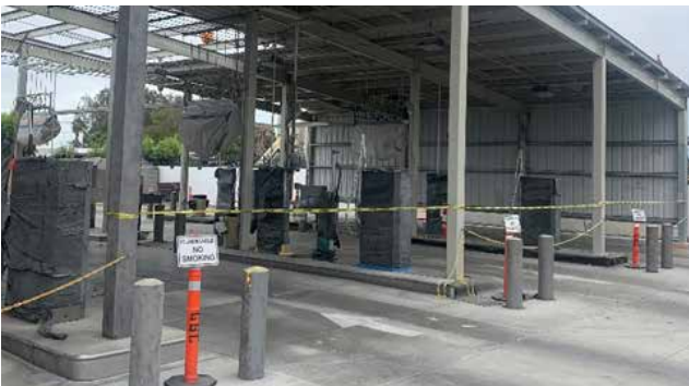
Oversaw building repairs at the Irvine Construction Circle Bus Base, including the roof, lighting, coatings, and structural work.
